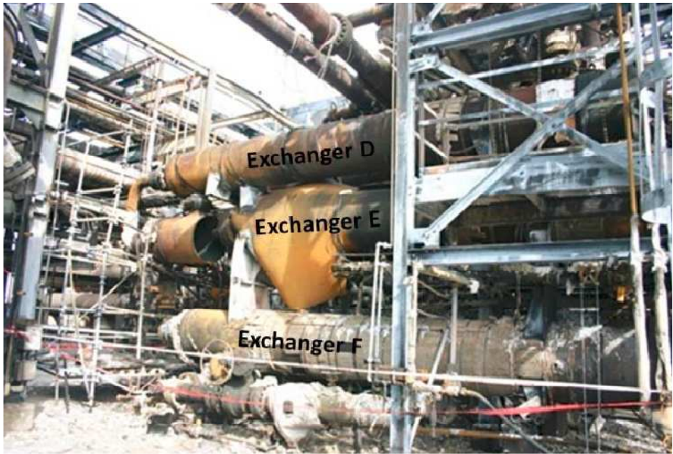
Figure 5: Post Incident View of the D/E/F NHT Heat Exchanger Bank
